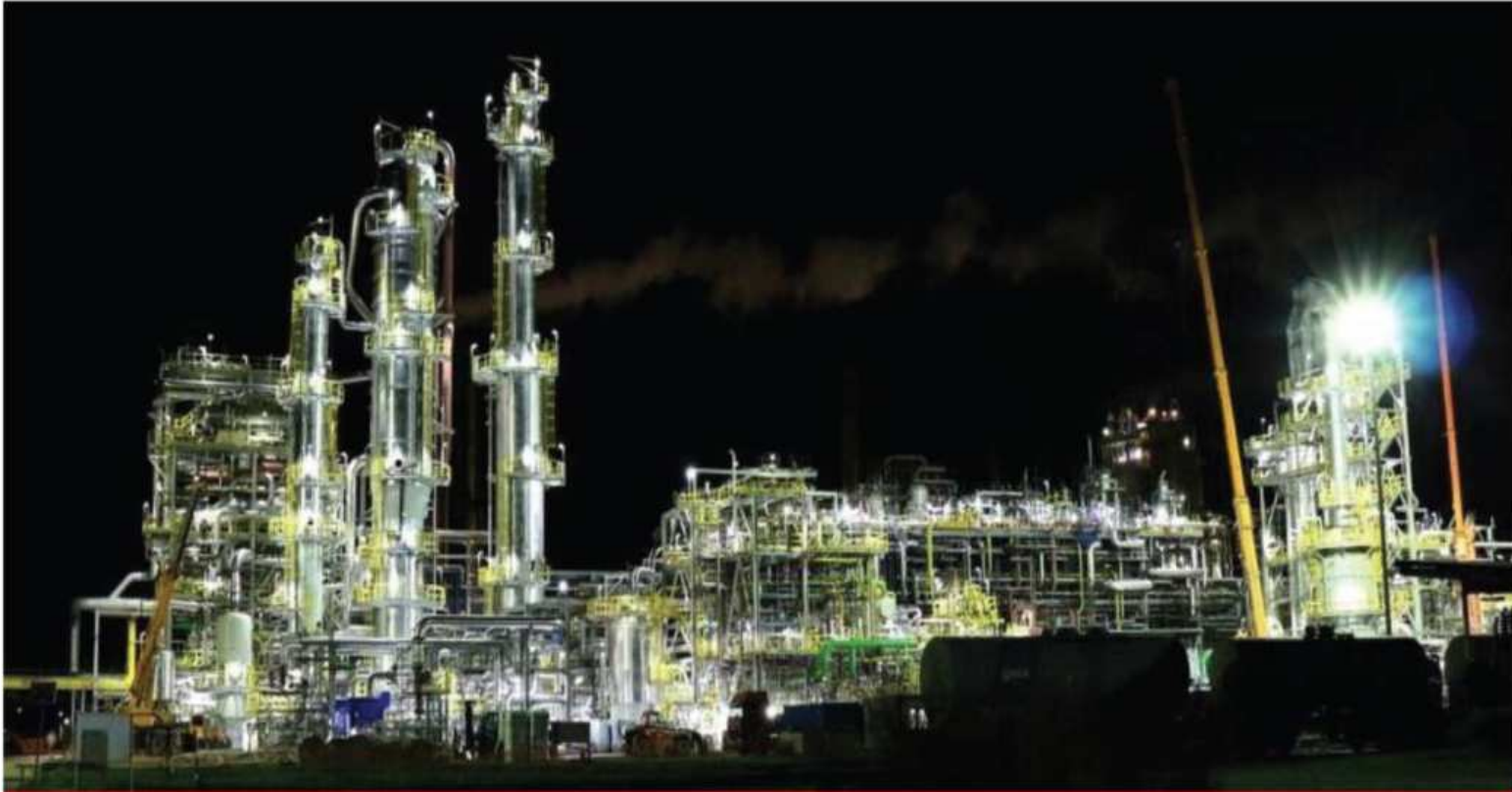
DUSLO PETROCHEMICAL PLANT - 1st TECHNIP'S WORLDWIDE PLANT FULLY EQUIPPED WITH HAZARDOUS AREA LIGHTINGS WITH LED SYSTEM (APPLETON TECHNOLOGY) SUPPLIED BY VIMEX
